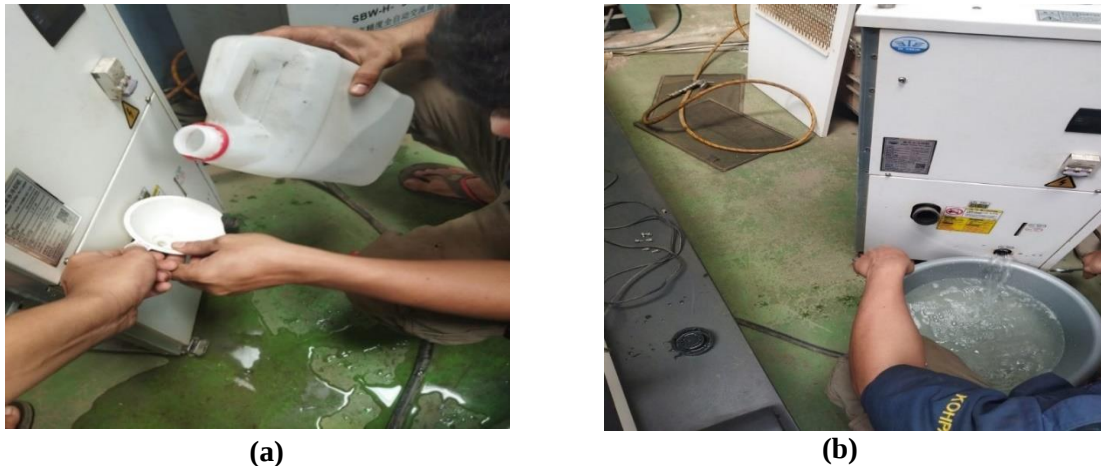
Gambar 6. Dokumentasi Preventive Maintenance Water Chiller
