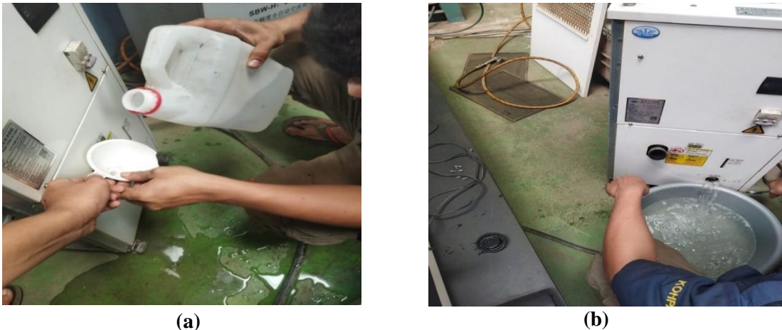
Gambar 6. Dokumentasi Preventive Maintenance Water Chiller
