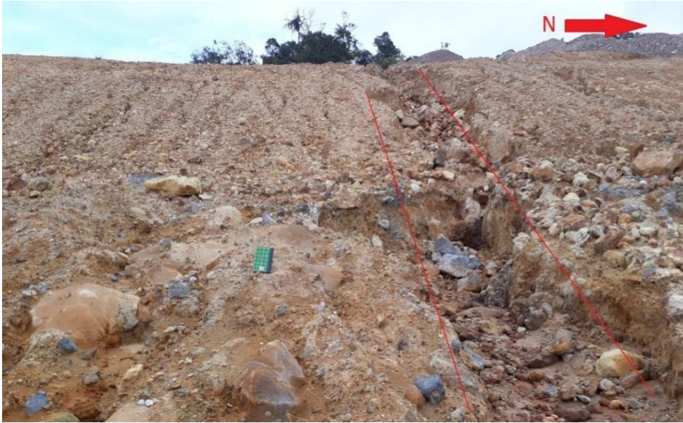
Figure 11. Field condition of water runoff flow in waste dump 1c
