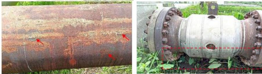
Figure 4. CUI indicates on the pipe in the X field [15]
